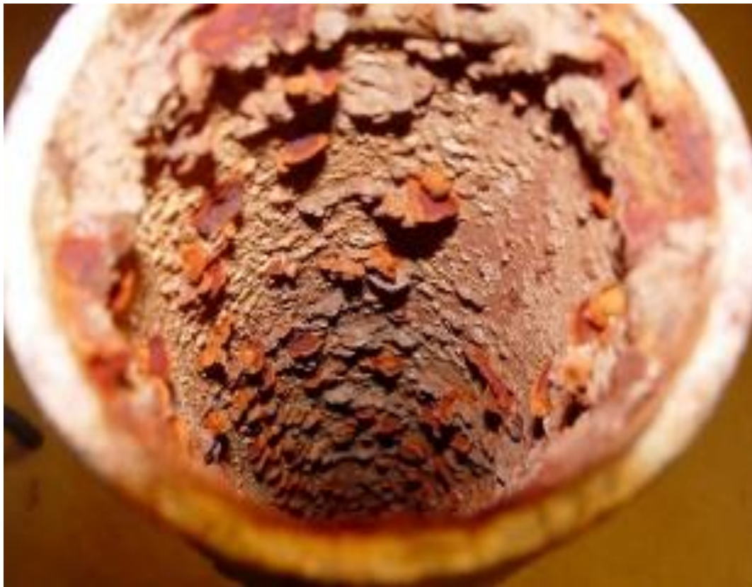
Plate 2.1: Corroded Metal Pipe (Adapted from Jerner, 2016)
